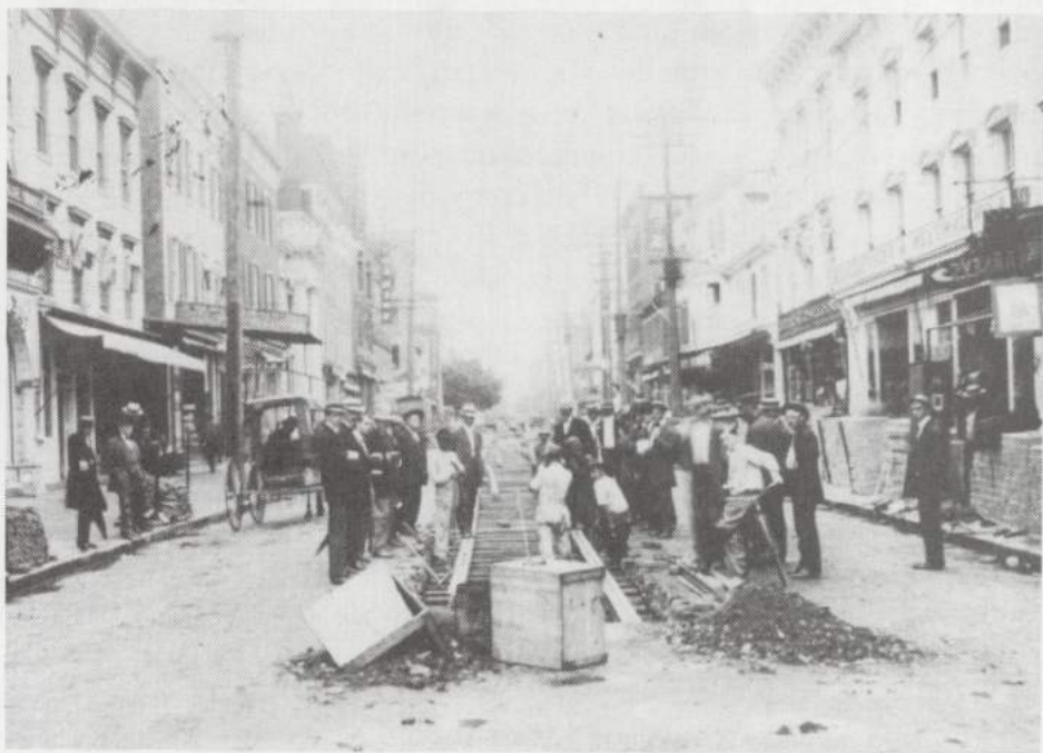
It was an exciting time when the trolley tracks were laid on North Market Street in Frederick! This part of the system was closed, and the tracks removed, in 1937.
