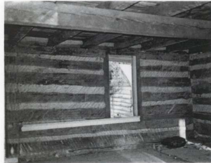
THIS PHOTO SHOWS THE INTERIOR OF "MORTALITY," THE HOME OF STEPHEN RAMSBURG, WHICH WAS STANDING ALONG ROUTE 15 FOR OVER 250 YEARS.
