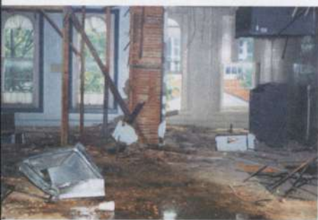
At the time the city of Frederick acquired the old Carty building, the structure was in significant disrepair and required major rehabilitation.
