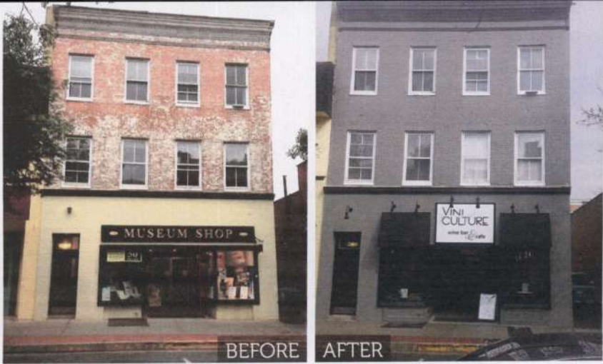
Downtown Frederick Partnership's Façade Improvement Program gives old buildings a fresh look.
